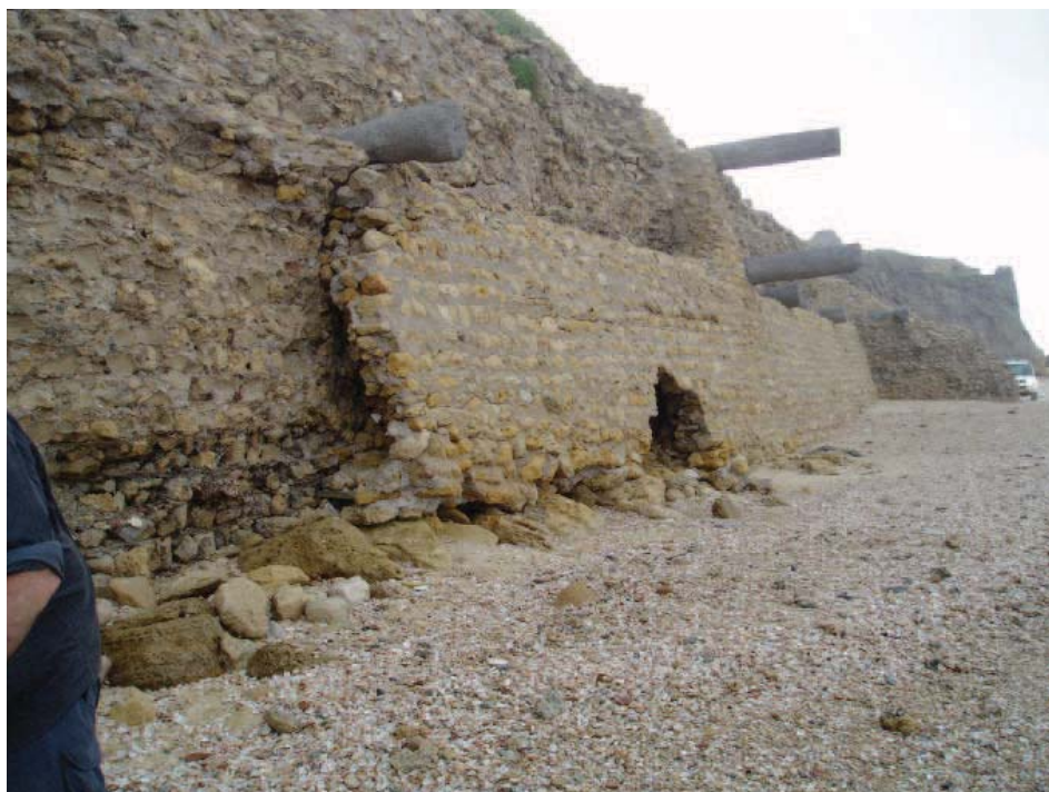
Figure 4 The Ashkelon seawall during 2012 after storms damage (G. Almagor).
