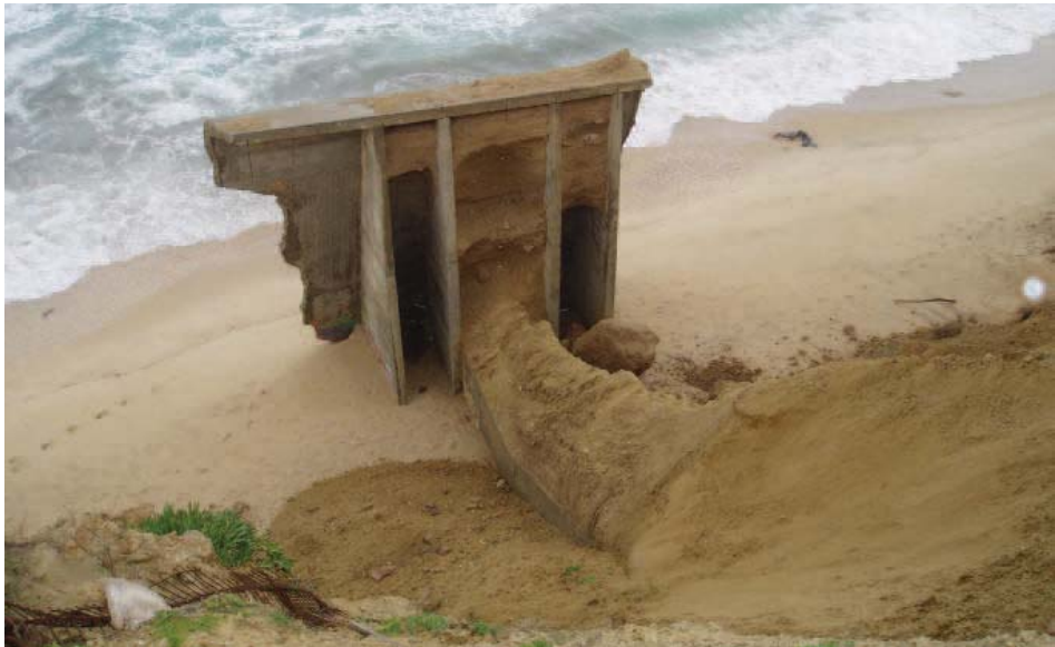
Figure 7. A drainage outlet on the Ashkelon north beach demonstrating coastal erosion of ca 15 m since 1999, when it was constructed (G. Almagor).
