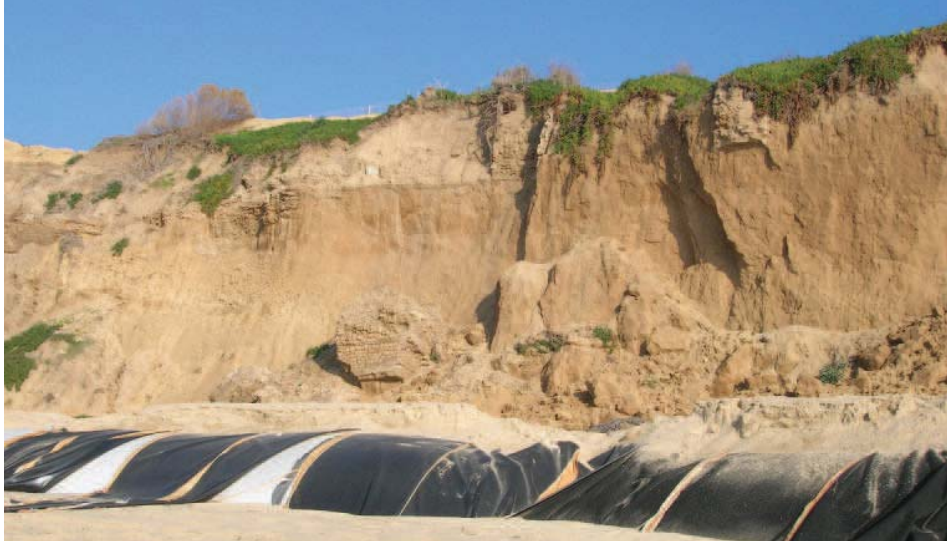
Figure 6. A collapse of the cliff and a monumental building on the Ashkelon north beach (E. Galili).
